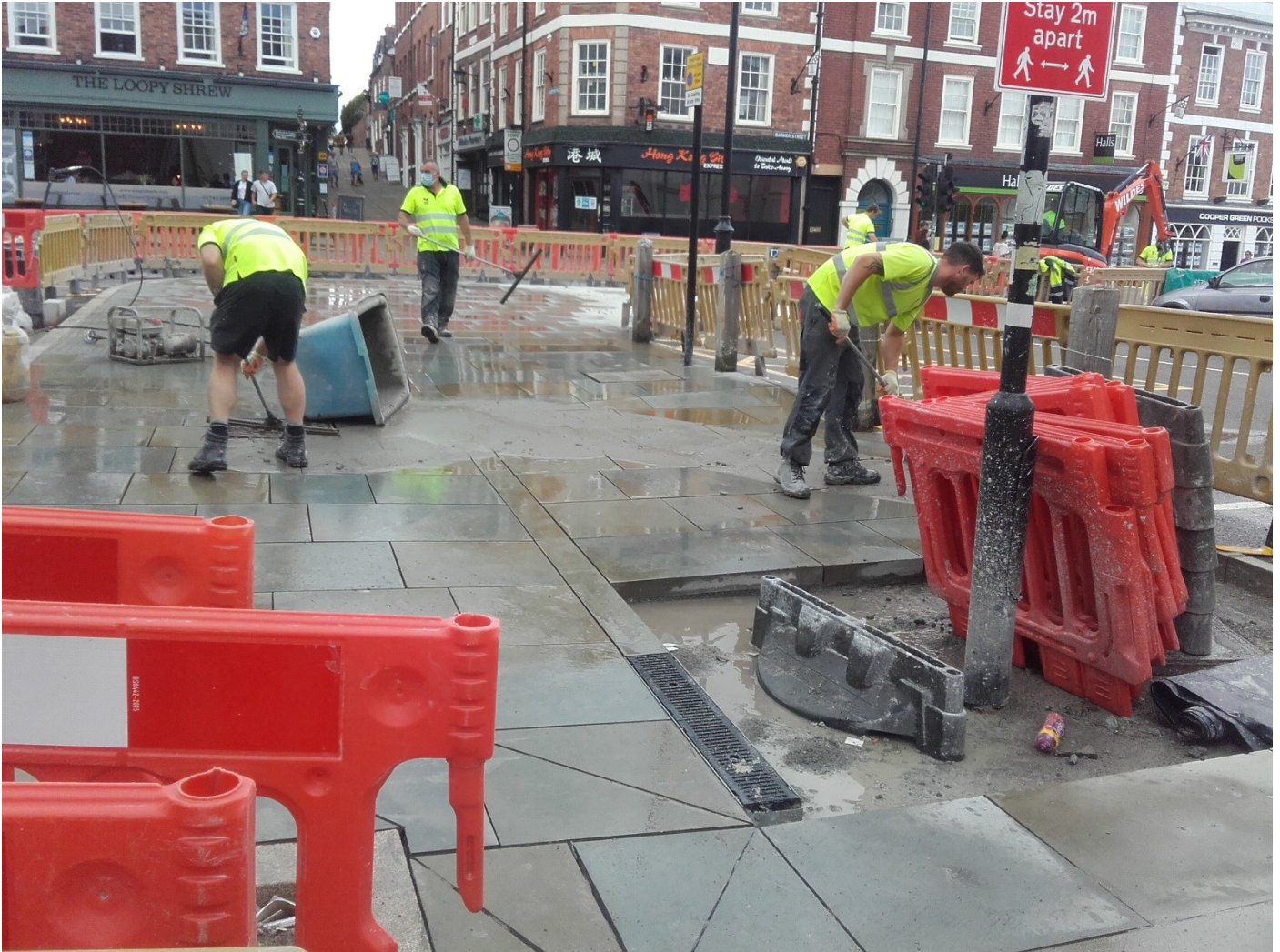
Grout being laid to joints of new Yorkstone paving on junction of Claremont Street into Barker Street
