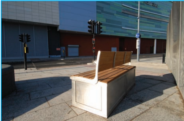
Bench containing traffic signal controller
